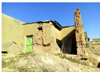
Fig 1 The effects of rainfall on exposed wall Source: Author's field photo archive. Nov 2017.
